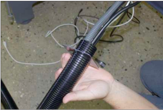
Figure 4-188: Loose end of corrugated tubing and all cords put through the access panel.
